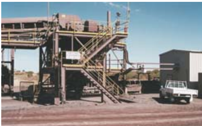
Conveyor plant drive unit
